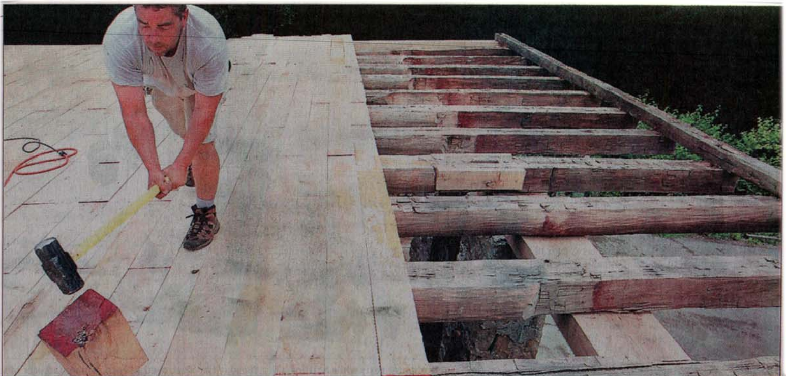
Brian Beals of Evolution Design/Build in Springfield uses a sledgehammer Tuesday to pound uneven spots in a rough-hewn floor of the barn that is being constructed at George Rogers Clark Park. Beals is one of two local instructors at the Timber Framers workshop, which is reconstructing the barn using a combination of original and new timber. The final raising of the barn is scheduled for Saturday. Staff photos by Barbara J. Perenic
