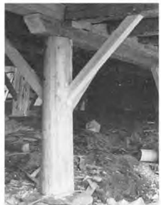
New cedar posts and braces under the Hadsell barn (c. 1860), St. Johnsbury, Vermont, a fully-functional repair.
