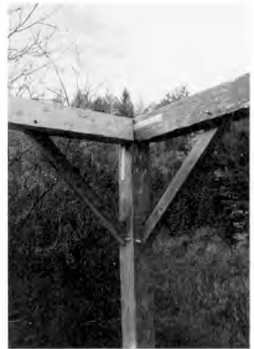
New hewn gable plate with free tenons fitted to post and eave plate, preserving most fabric. Bean barn (c. 1820), Barnet, Vermont.
