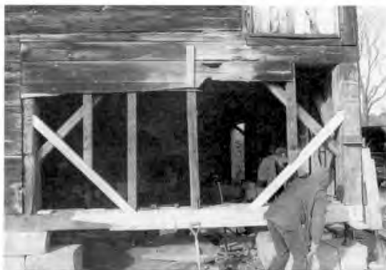
Sill and brace restoration by Paul Ide and Don Estes. Note jacking plate on corner post. Foundation to be restored. Kent Barn (1844), Calais, Vermont.
